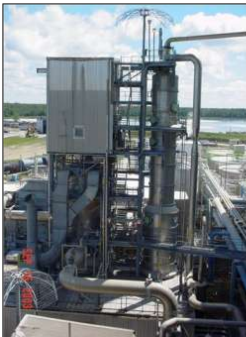
Figure 30 Commercial Booster plant at New Bern
